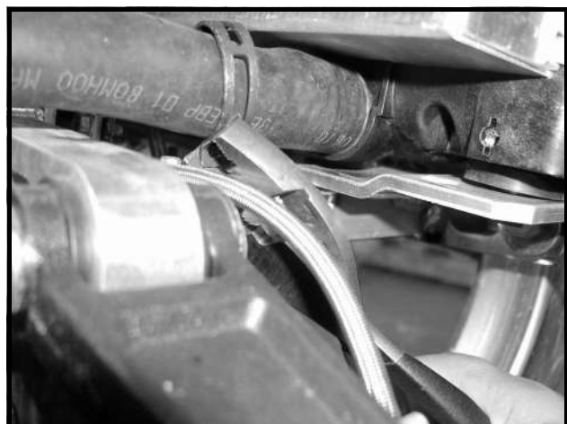
Figure 15-3 Reservoir Outlet Hose
