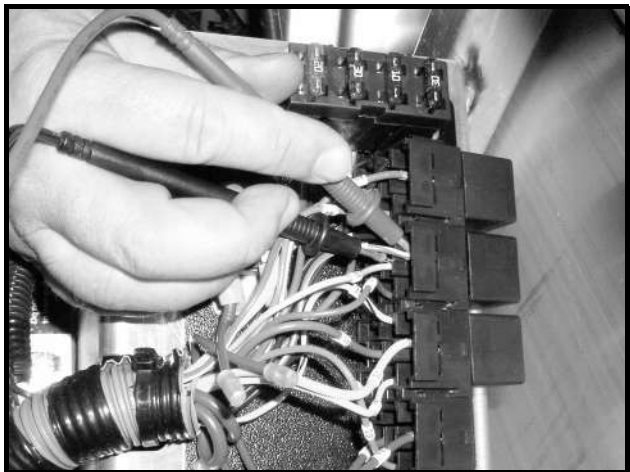
Figure 11b-14 Differential Relay Contact Test
