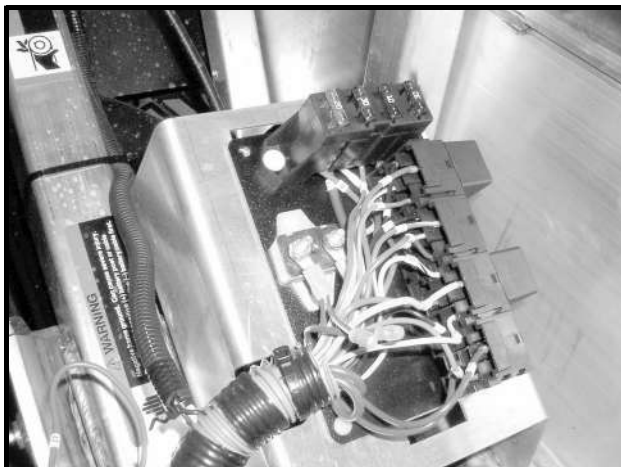
Figure 11b-24 Differential Relay Removed
